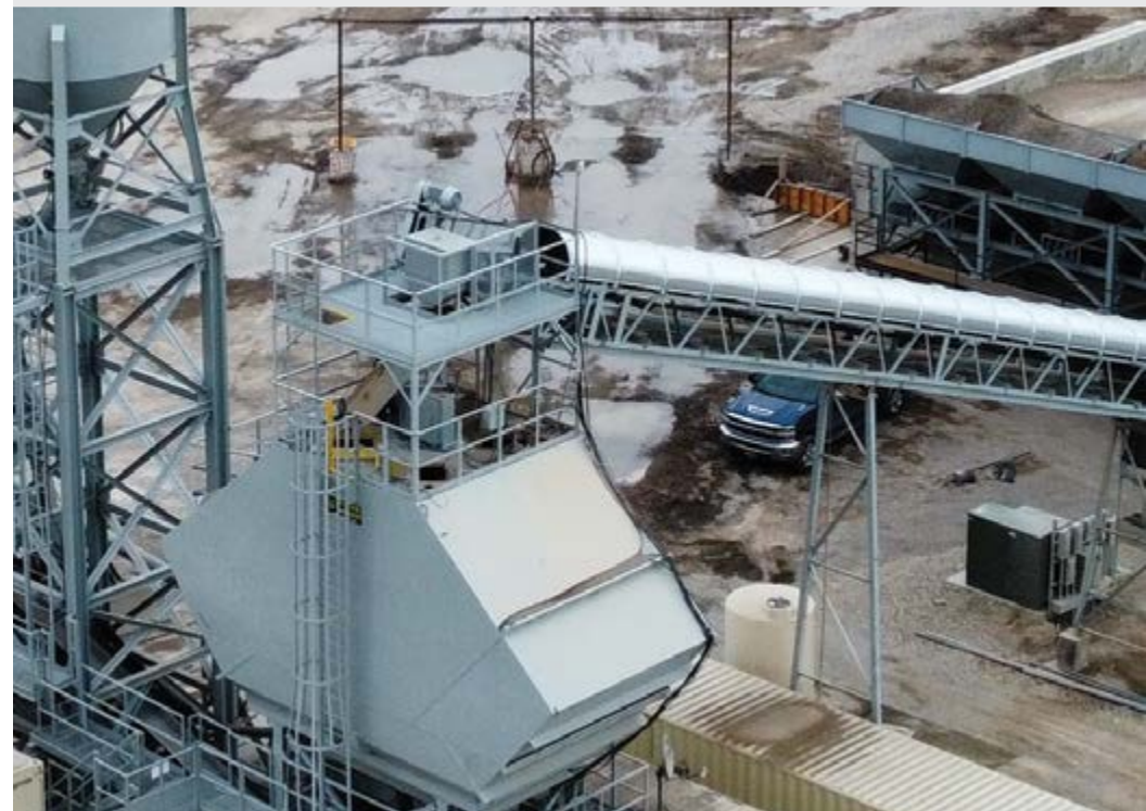
STATIONARY CONVEYOR WITH TURN HEAD
