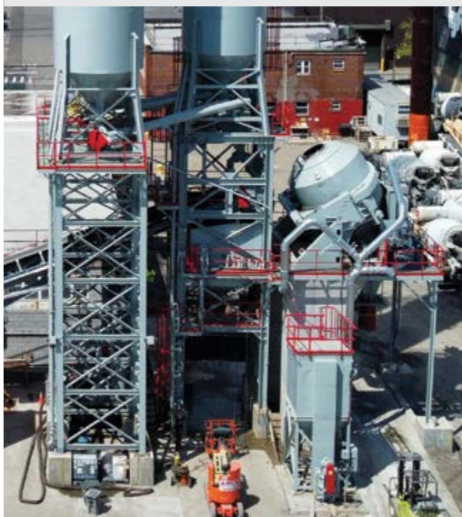
DUAL LANE (DRY & WET) LPM PAIRED WITH 12 YD 3 STATIONARY TILT MIXER
