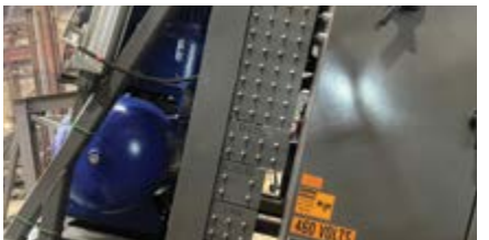
CENTRALIZED GREASE STATION
