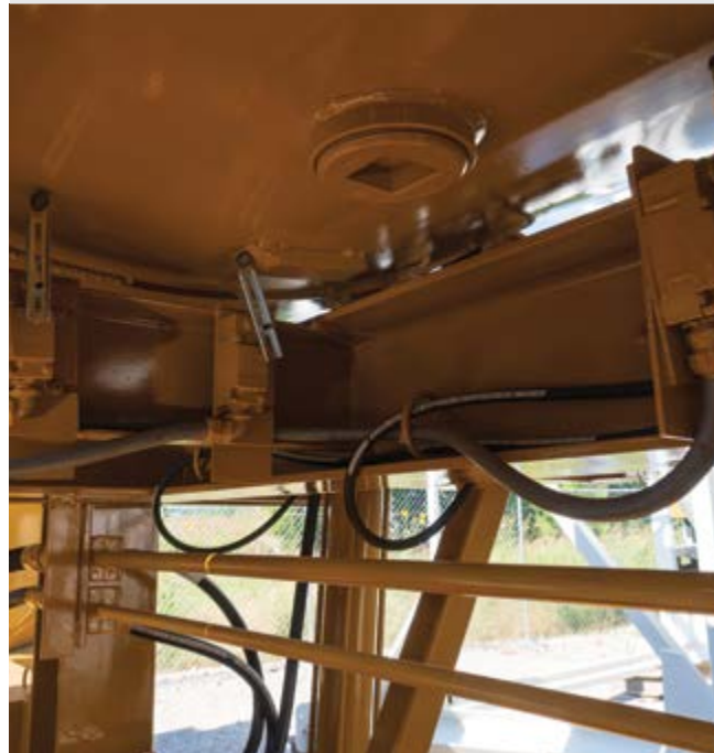
LIMIT SWITCHES FOR TITLED, RETURNED, EARLY RETURN TO SPEED LOADING PROCESS
